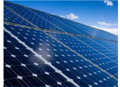
Solar power systems
